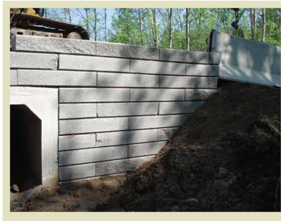
This amphibian culvert crossing currently under construction in Guelph, Ontario demonstrates the type of creative problem solving that often is not in our mindset when we think about our public infrastructure.
